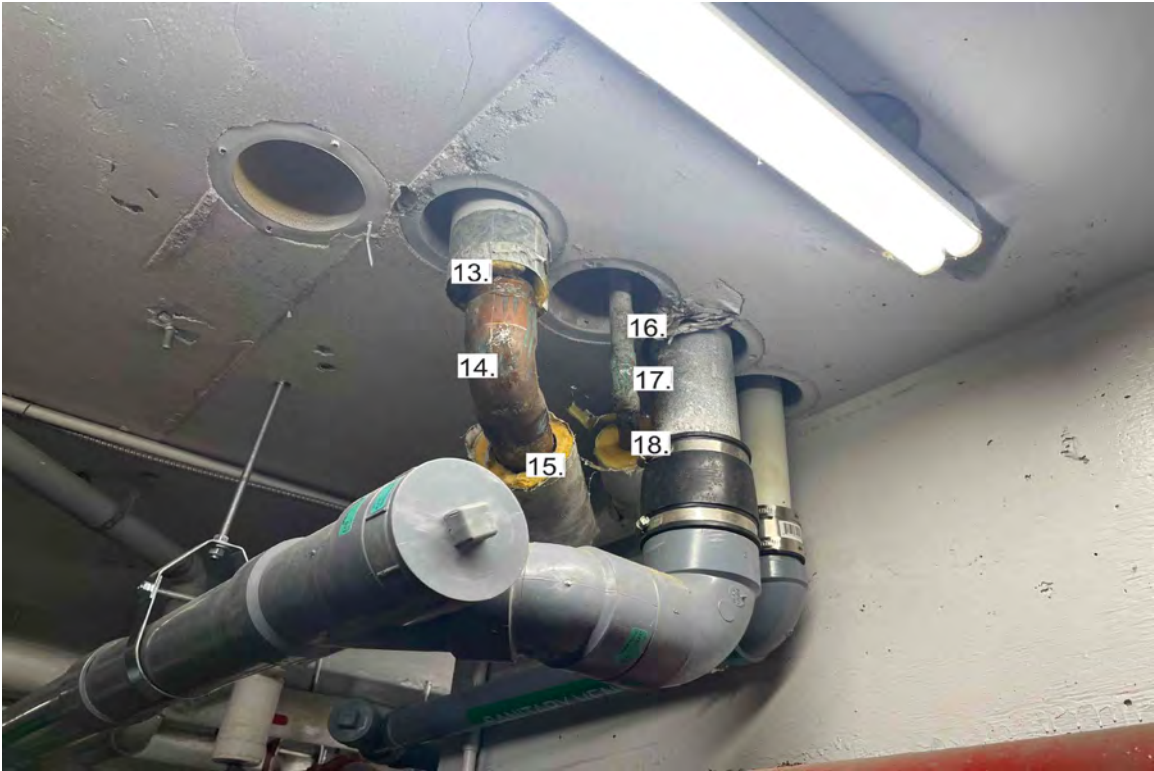
Photograph 3: Parking Garage Spot #6.
