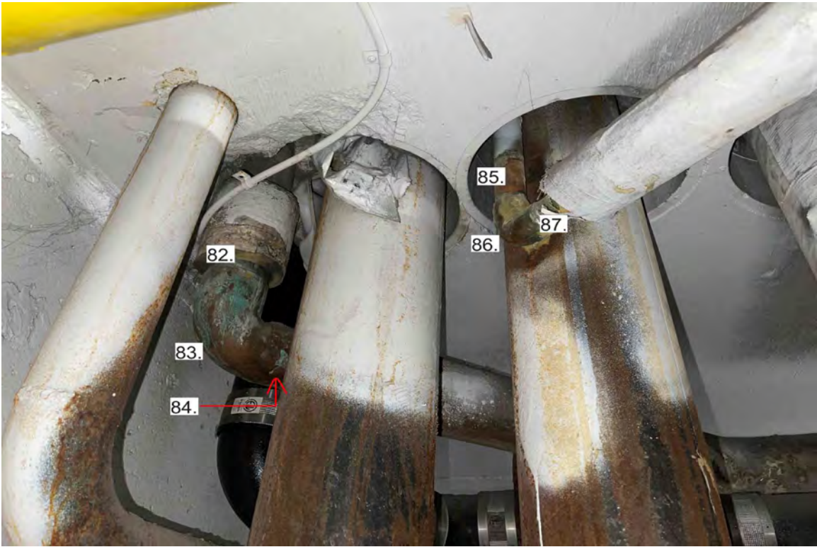
Photograph 15: Parking Garage Spot #19.
