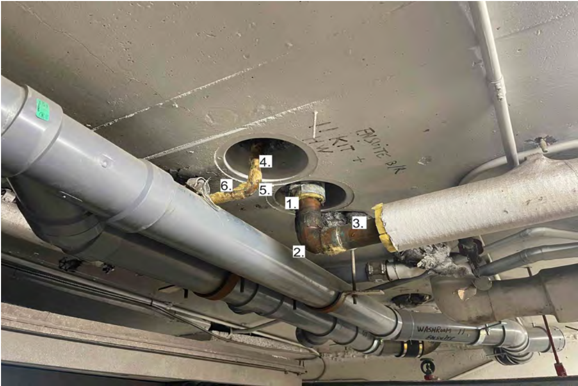
Photograph 1: In Front of garage door on level 1.
