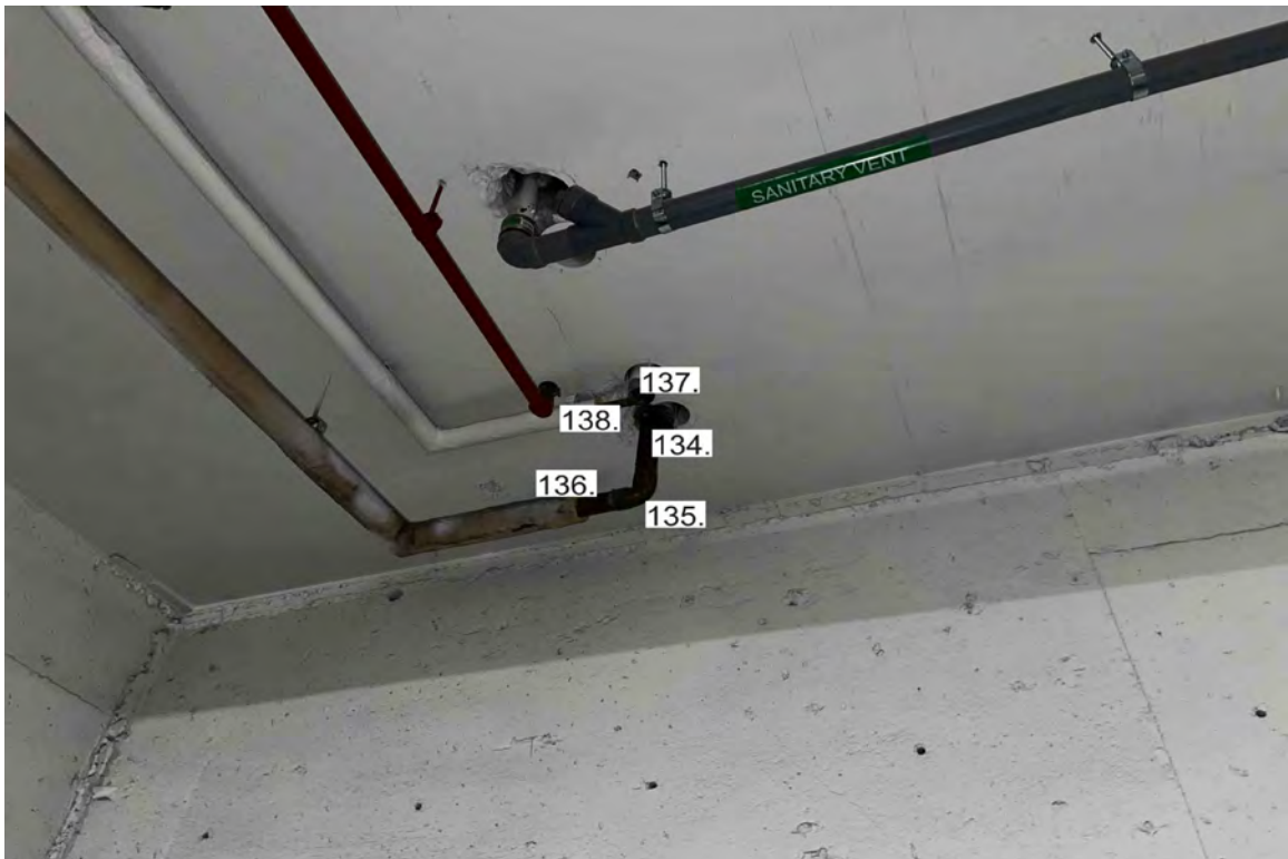
Photograph 24: Parking Garage Spot #1.
