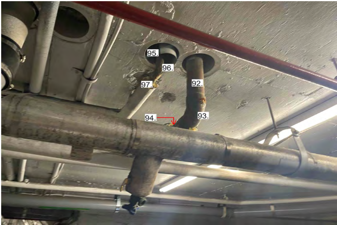
Photograph 17: Parking Garage Spot #21.
