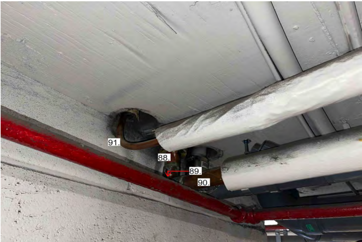
Photograph 16: Parking Garage Spot #20.
