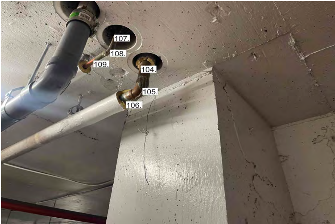
Photograph 19: Parking Garage Spot #24.
