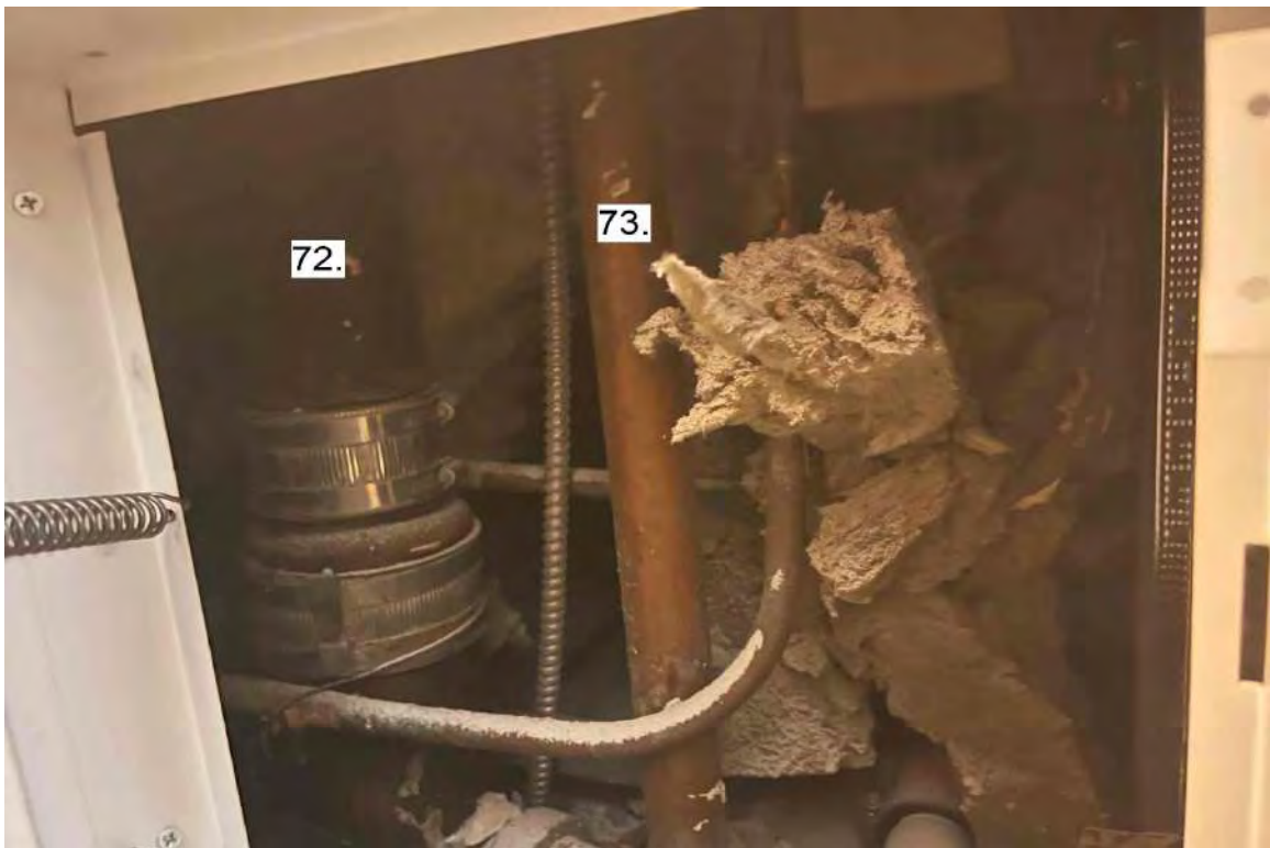
Photograph 38: 3 rd Floor Bathroom Stack Unit 302.
