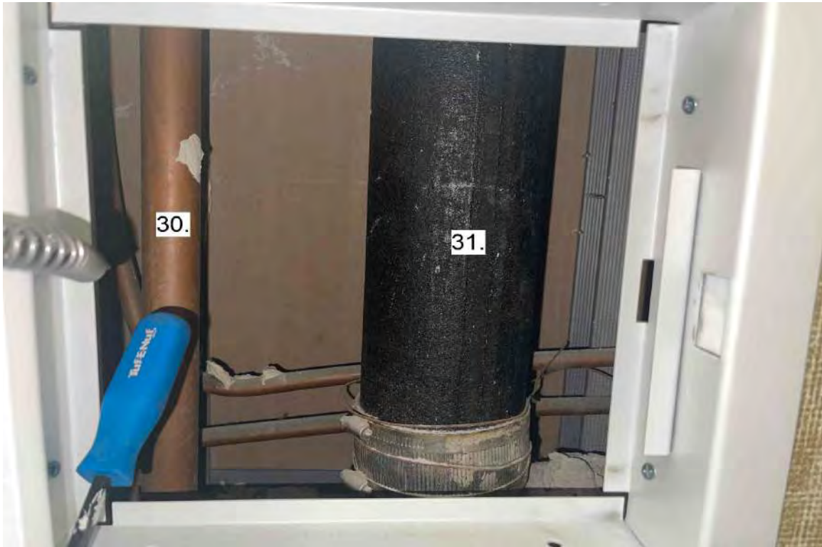
Photograph 16: 9 th Floor Bathroom Stacks Between Units 903 & 902.
