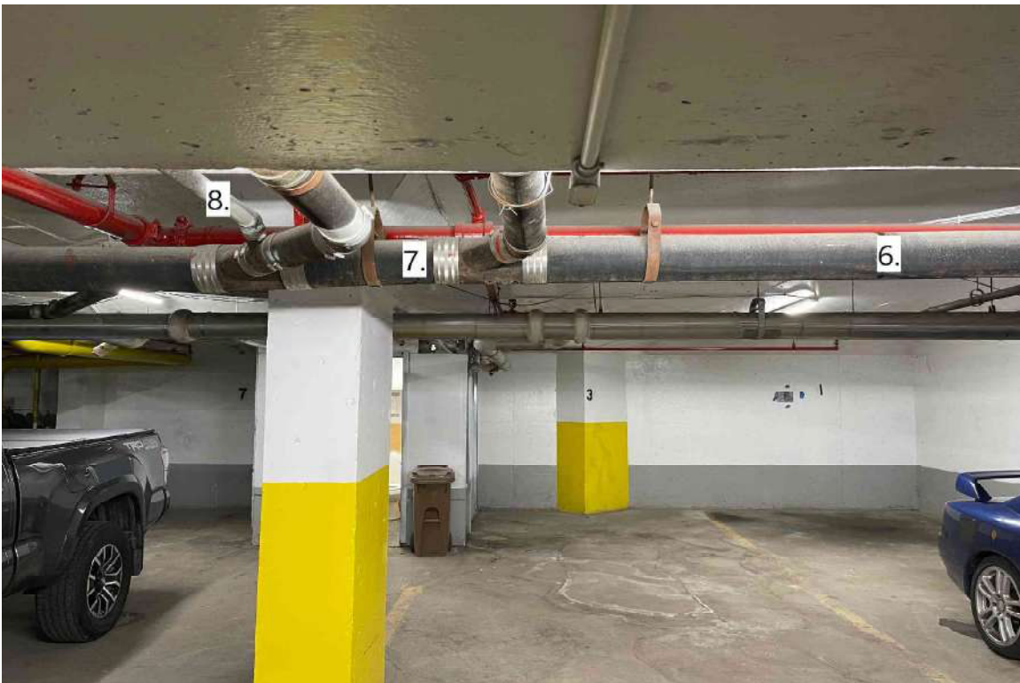
Photograph 2: Parking Garage Spot 3.
