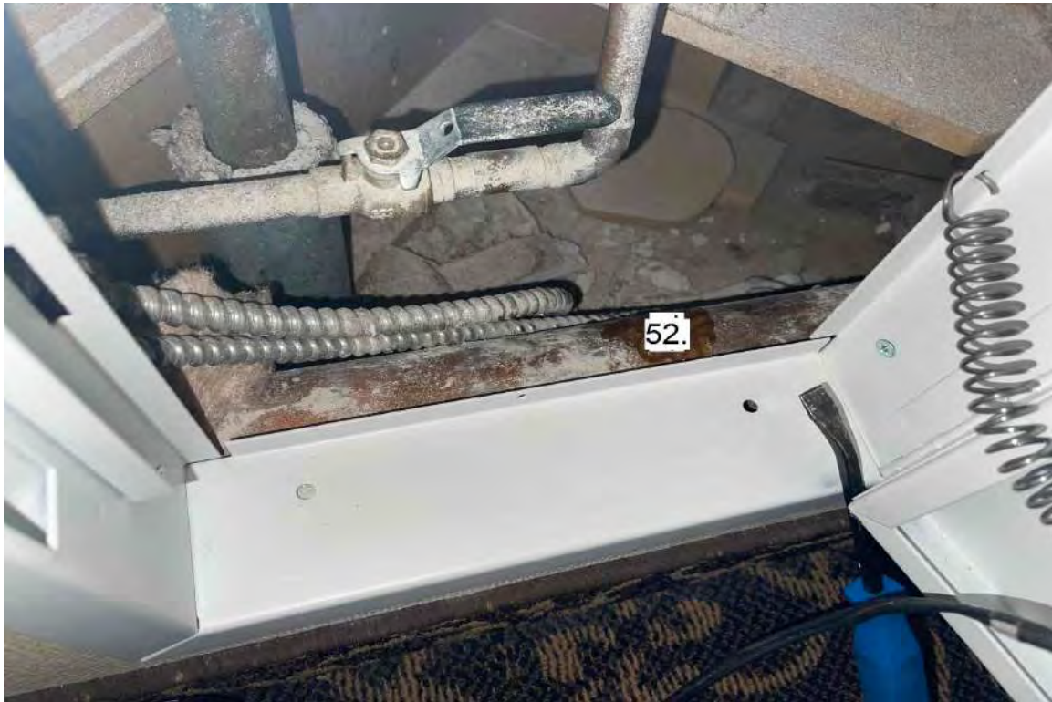
Photograph 27: 6 th Floor Bathroom Stack Between Units 607 & 608.
