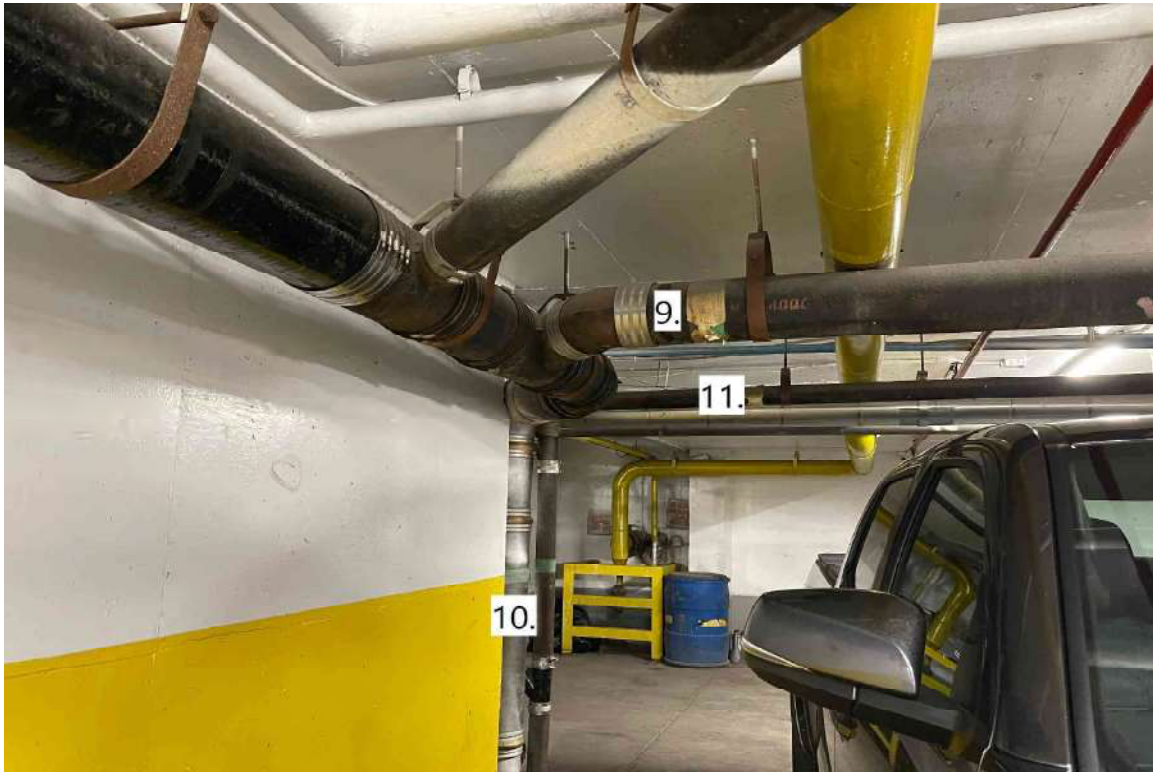
Photograph 3: Parking Garage Spot 7.
