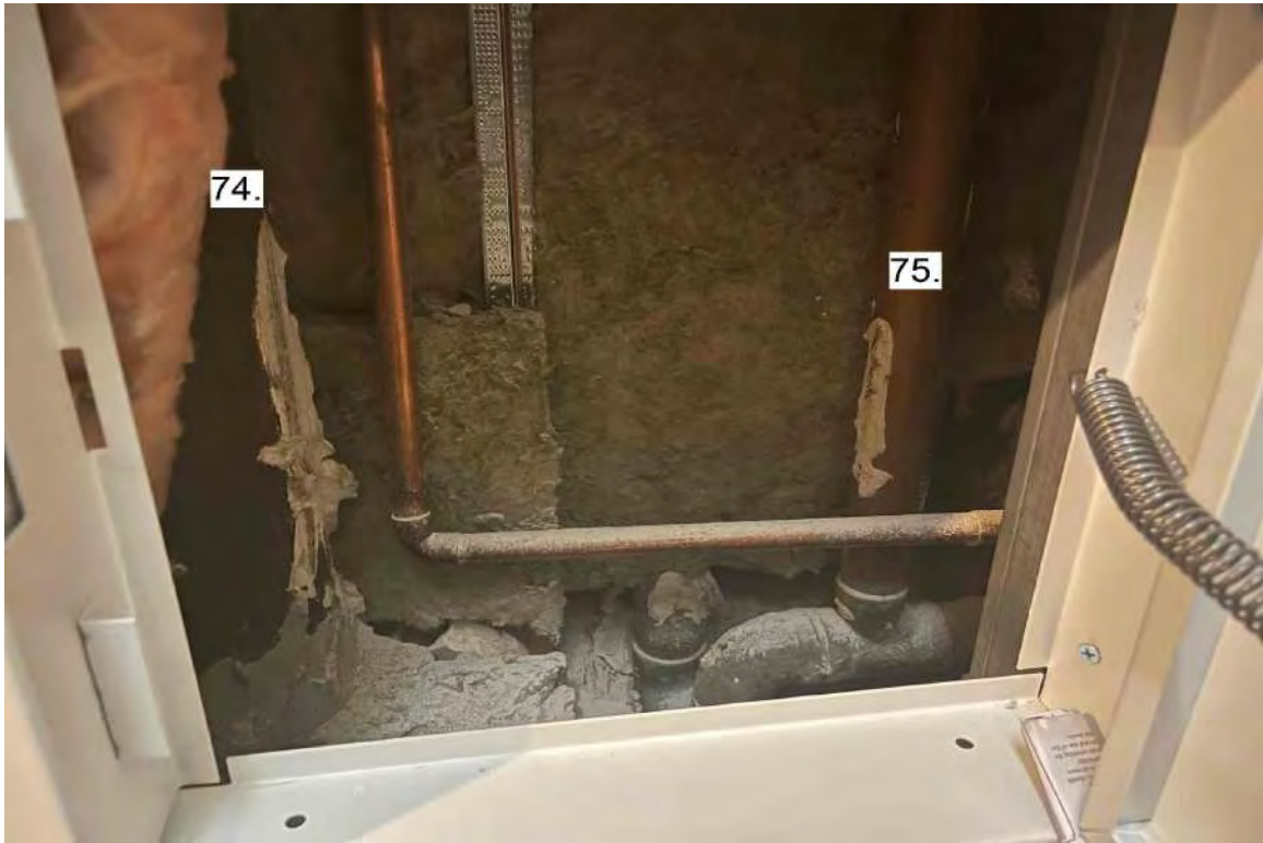
Photograph 39: 3 rd Floor Bathroom Stack Unit 302.
