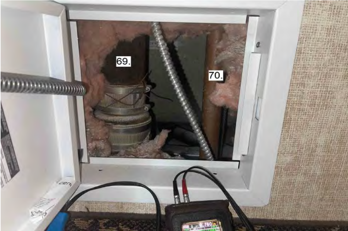
Photograph 36: 3 rd Floor Bathroom Stack Unit 307.
