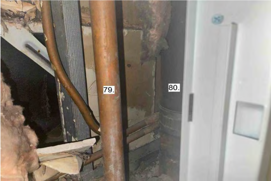
Photograph 42: 2 nd Floor Bathroom Stack 1st Hatch Unit 206.
