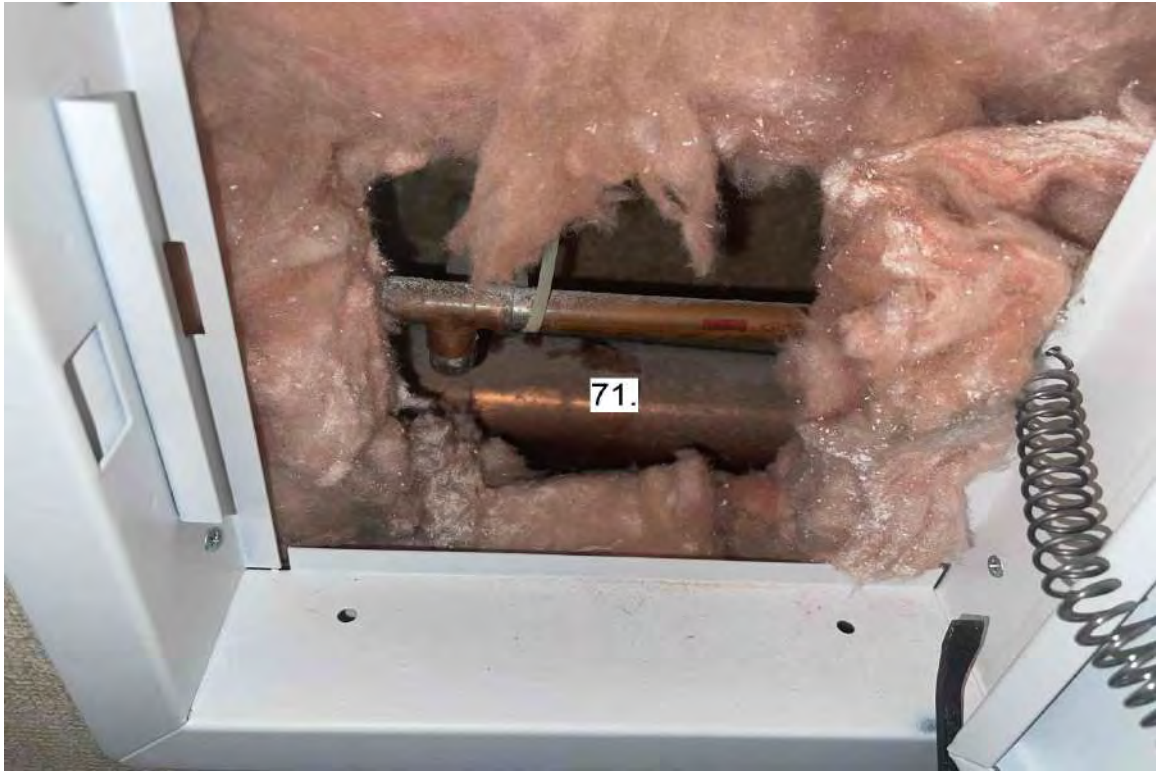
Photograph 37: 3 rd Floor Bathroom Stack Unit 307.
