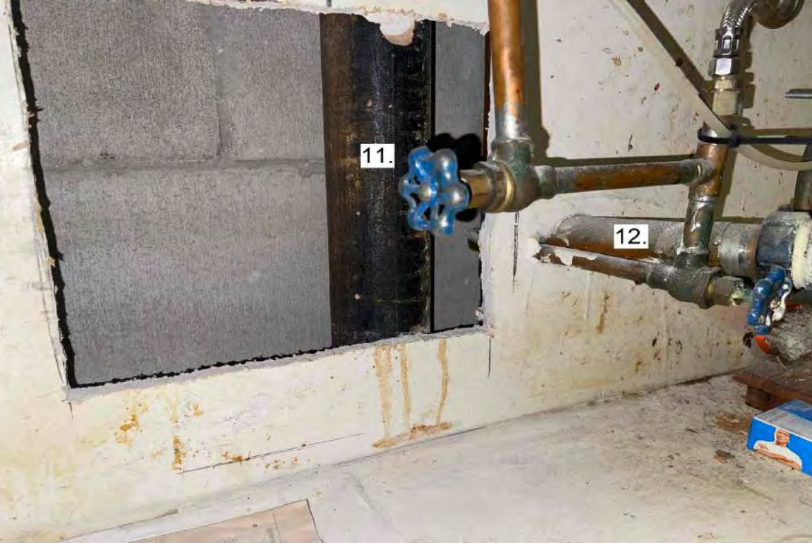
Photograph 6: 7 th Floor Unit 702.
