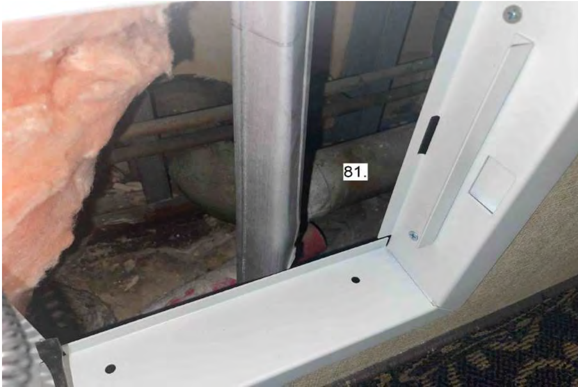
Photograph 43: 2 nd Floor Bathroom Stack 2 nd Hatch Unit 206.
