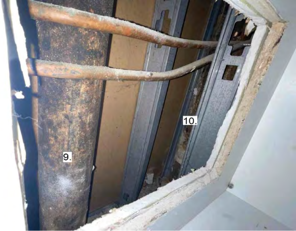
Photograph 5: 7 th Floor Unit 701.
