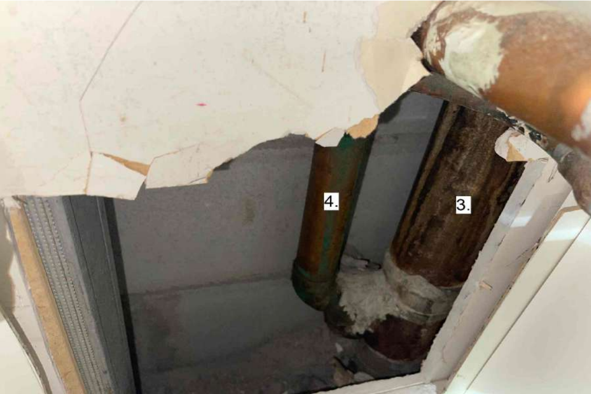
Photograph 2: 11 th Floor Unit 1108.
