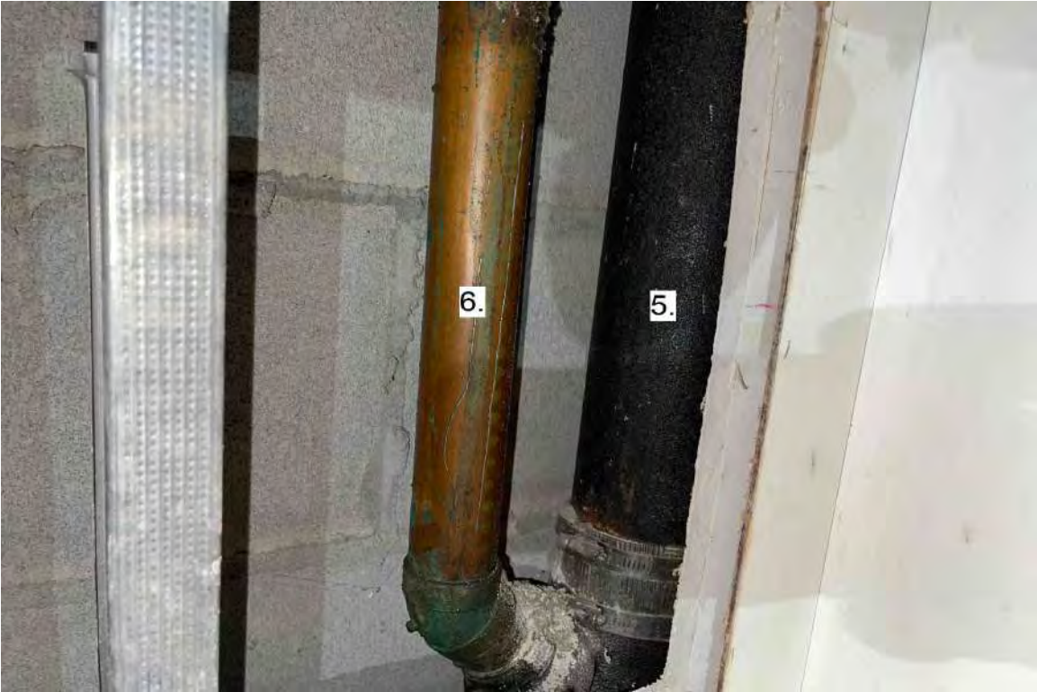
Photograph 3: 11 th Floor Unit 1105.
