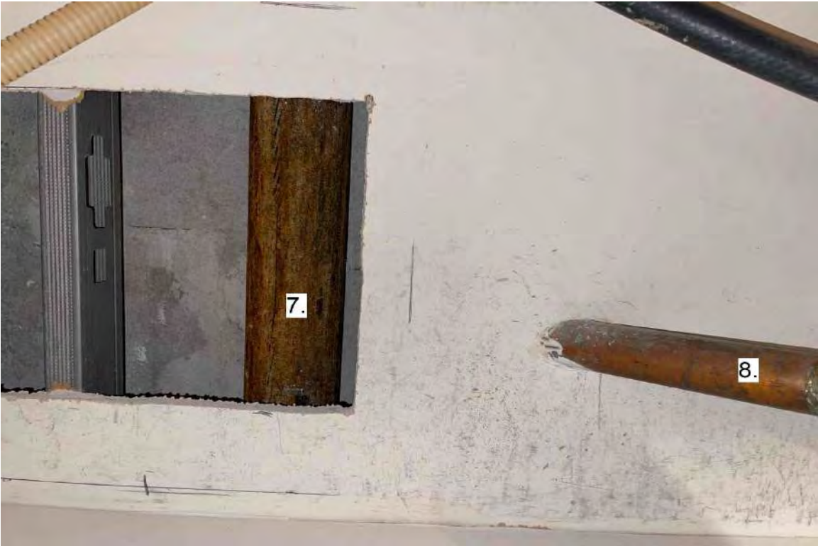
Photograph 4: 7 th Floor Unit 707.
